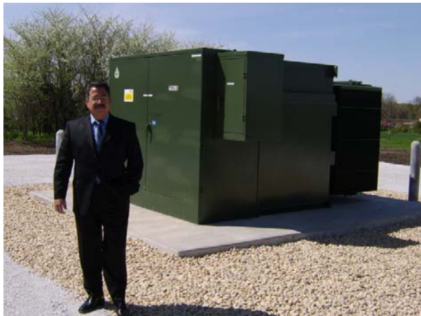
Substation in a box
